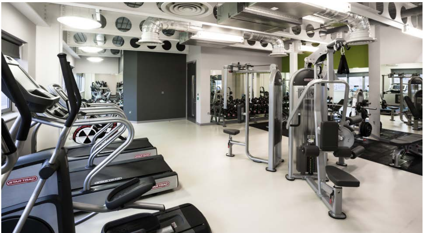
See overleaf for a few images of recent corporate gym installations we have completed.
